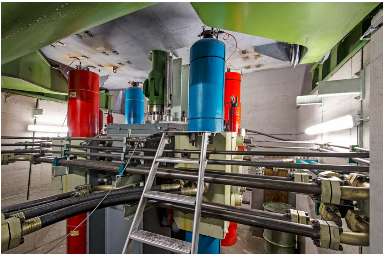
Main cylinder unit of the vertical shock test rig (VESPA).
